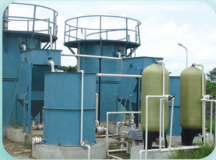
SAFF/MBBR/FAB SEWAGE TREATMENT PLANTS
