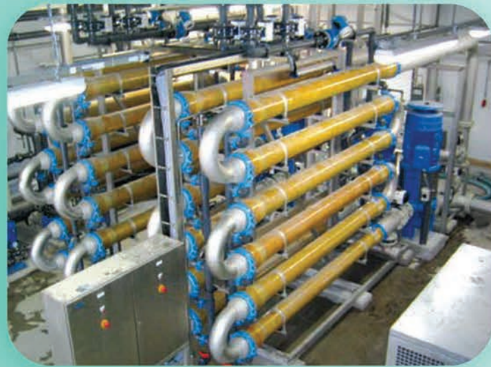
MBR WASTE WATER TREATMENT / ULTRA FILTRATION
